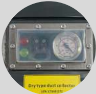
Filter clogging indicator and vacuum gauge with warning light
