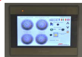
CONTROL PANEL BOARD WITH HMI DISPLAY ON DHV LINE
